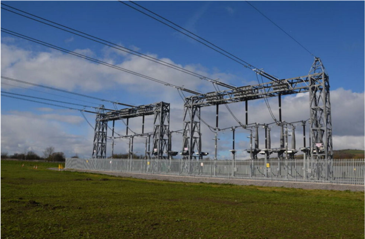
Image 3.9 Existing CSE compound with gantries (Source: ES Chapter 4: Project Description (document reference 6.4))
