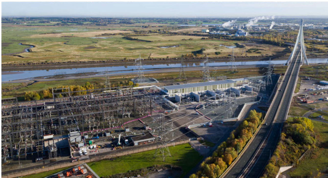
Image 3.3 Existing Connaught's Quay 400 kV Substation in colour cladding (Source: National Grid)
